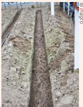
In mounds, the crowns are deposited about 20 cm deep, but at least 5 cm above the soil warming system.
